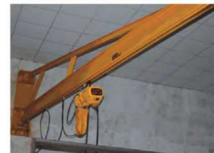
悬臂吊 Jib Crane
